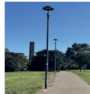
LP: Light pole
